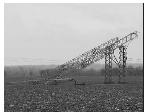
Signifying the storm's power, this transmission tower was toppled.
