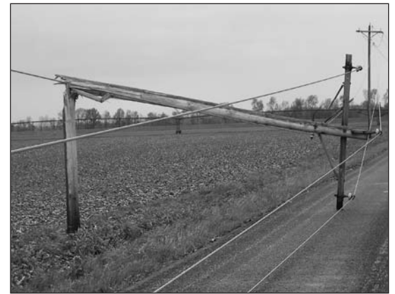
The severe storm caused significant damage to numerous poles in our service territory.
